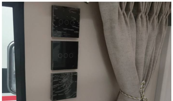
Fig. 3-3 Main Control Switch
